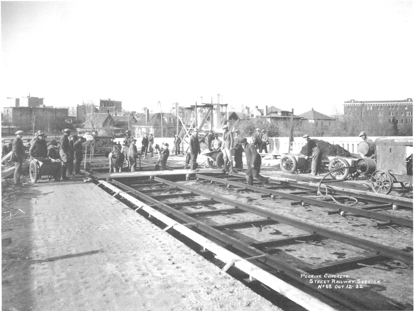
The Broadway Bridge under construction, October 1932. This was the largest unemployment relief work scheme completed in Saskatoon as part of the 1931-1932 shared cost program. Saskatoon Public Library, Local History Room. A-202
